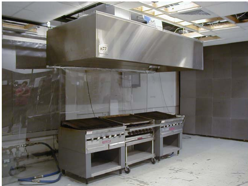
Figure 1. Halton KVE Wall-Mounted Canopy Hood Test Setup (Note Transparent Back Wall)
