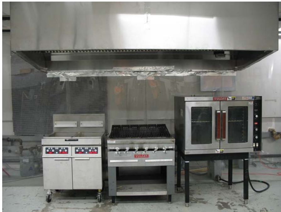
Figure 10. Fryer/Broiler/Convection Oven Appliance Line
