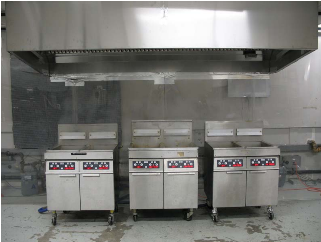
Figure 8. Medium-Duty Gas Fryer Line
